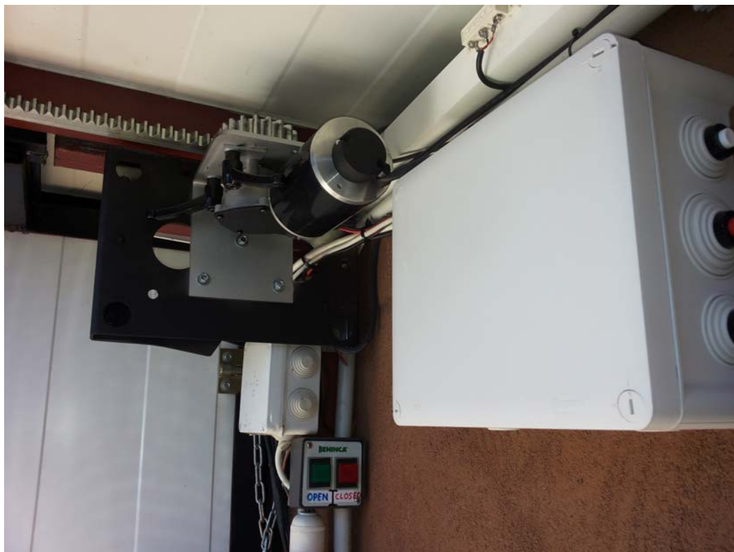
Talon6 installed in the left roof of the observatory
