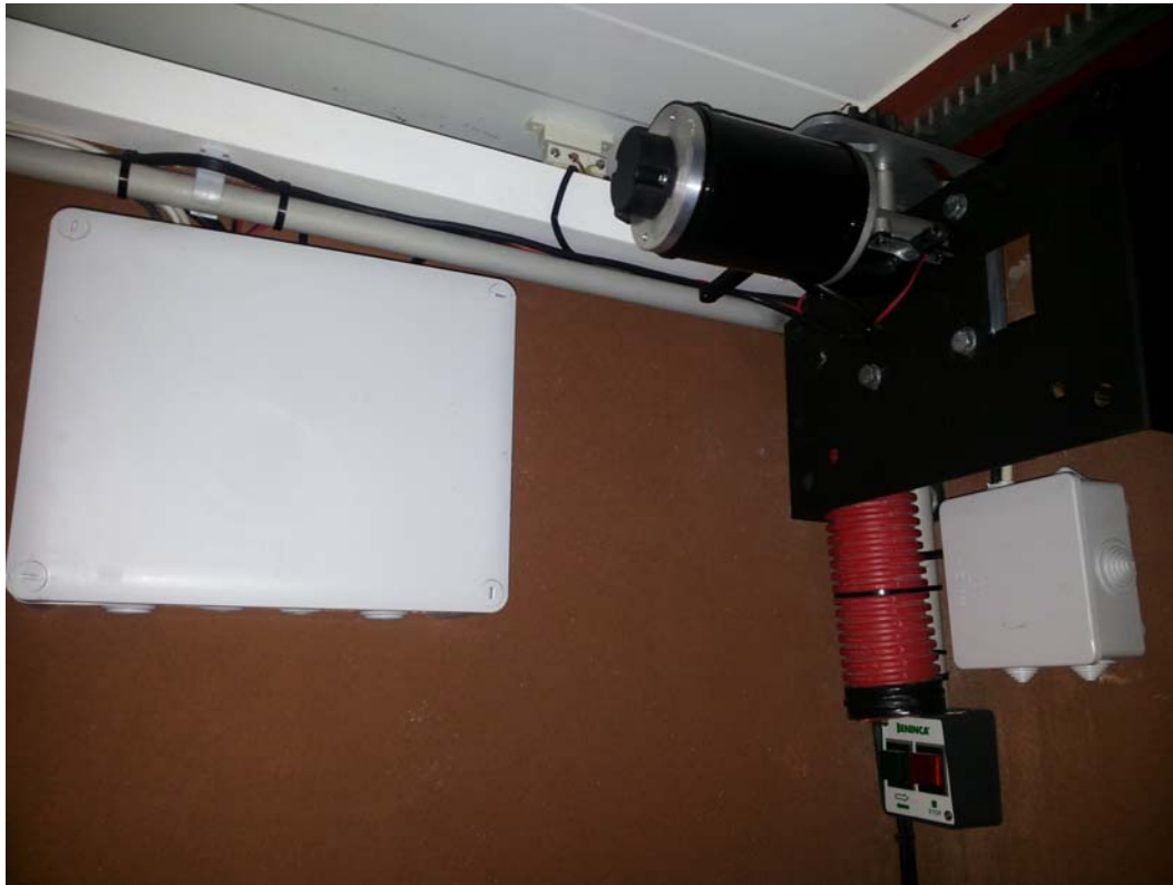
Talon6 installed in the right roof of the observatory
